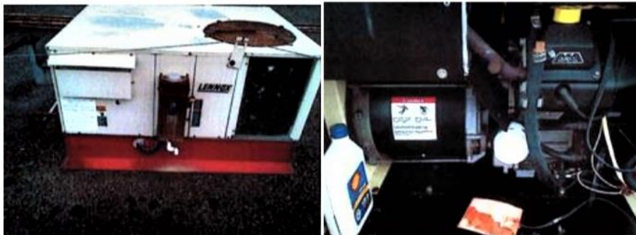
Current HVAC units are at the end of service life
