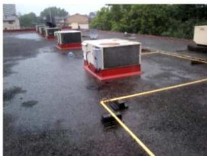
Current six HVAC units located on the roof
